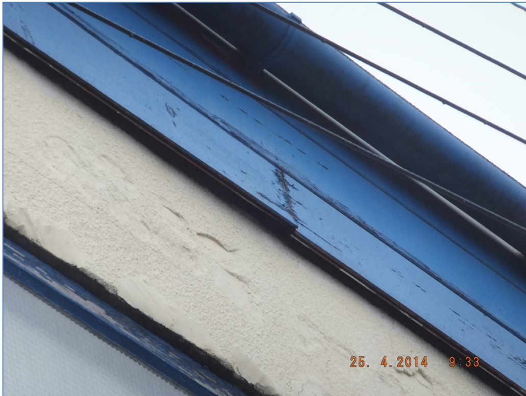
Photograph 5 Gaps under wooden cladding
