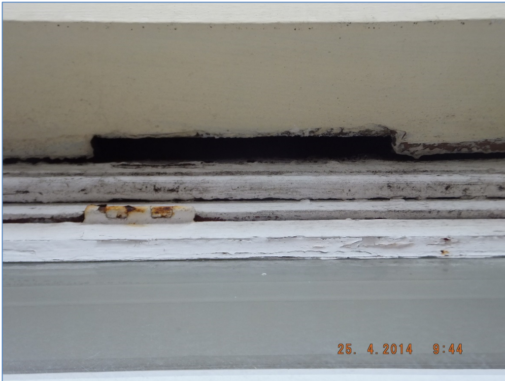
Photograph 3 Gap around windows
