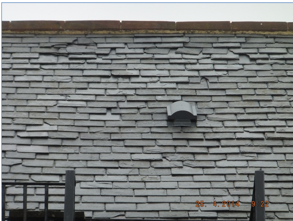
Photograph 2 Gaps under slates
