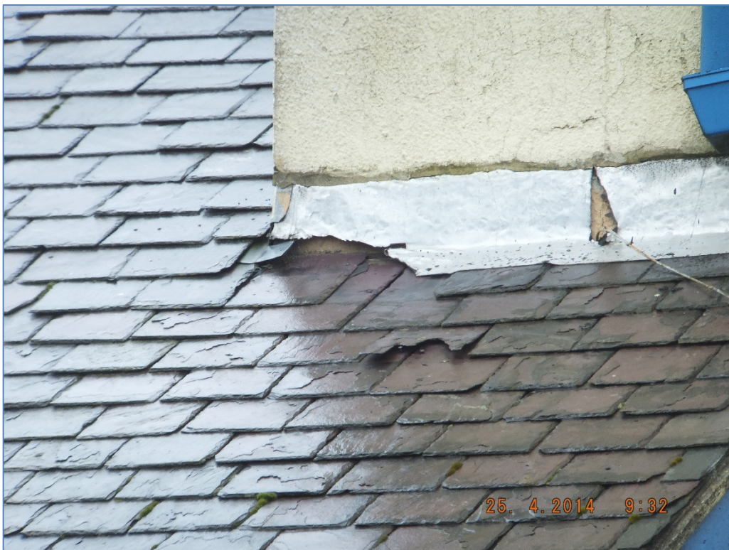
Photograph 4 Gaps under flashing
